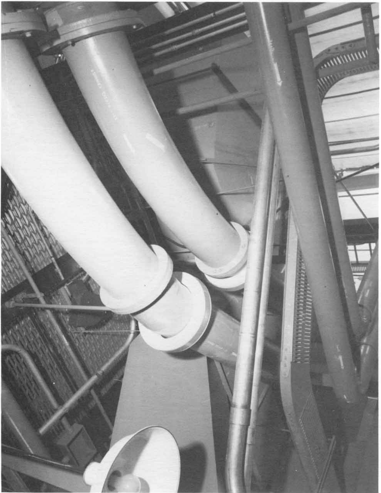
Twelve-inch diesel exhausts and ducting, looking up from elevator toward Column F (Neg. No. 68022A dated 4-26-61).
