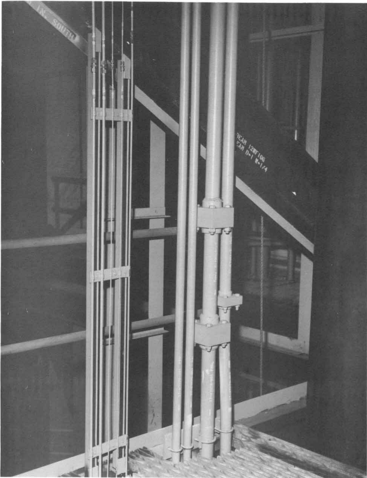
Vertical run, showing hydraulic pipes running through Level 4 (Neg. No. 67563A dated 4-19-61).
