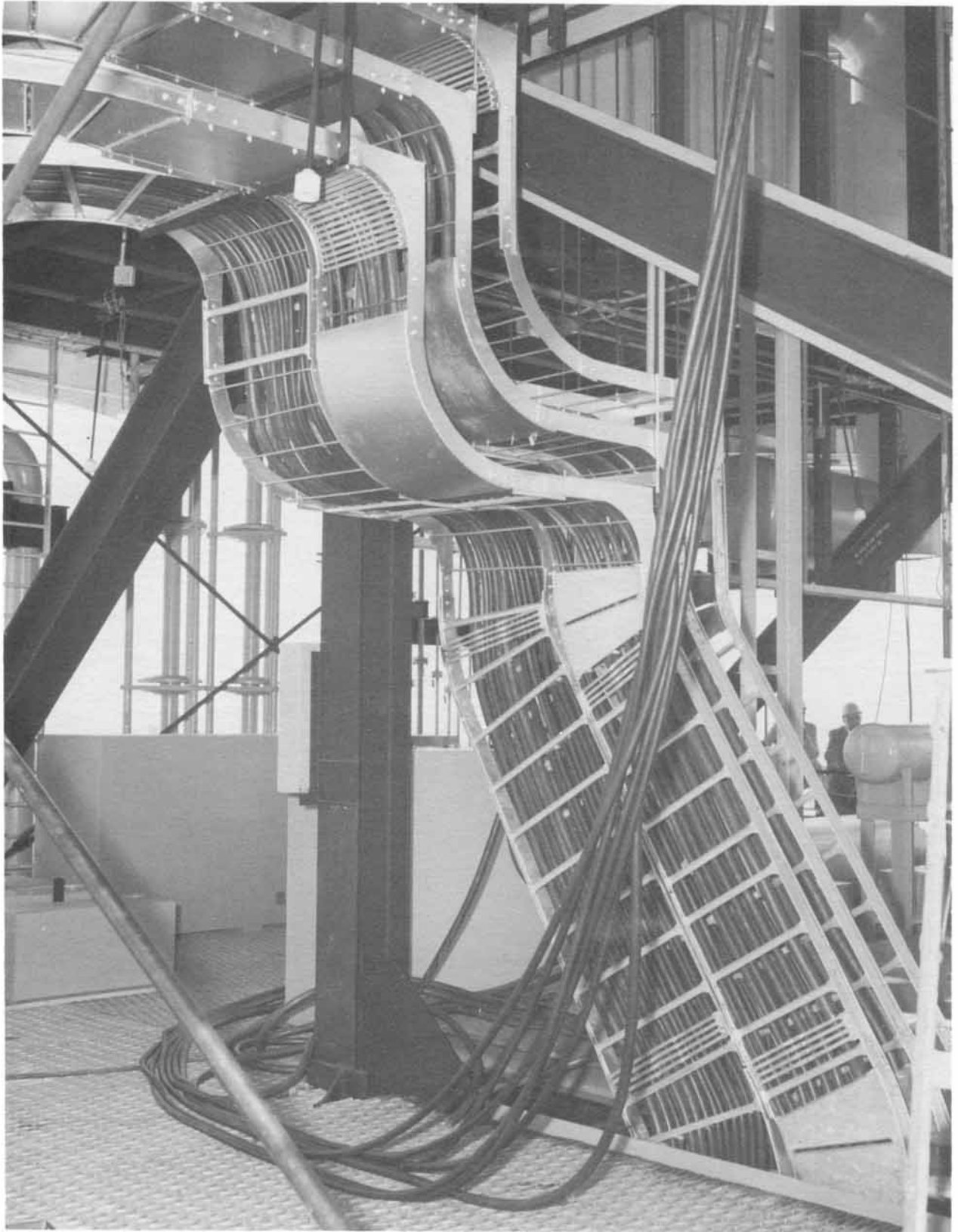
Cable trays on Level 4 (Neg. No. 53295A dated 8-8-60).
