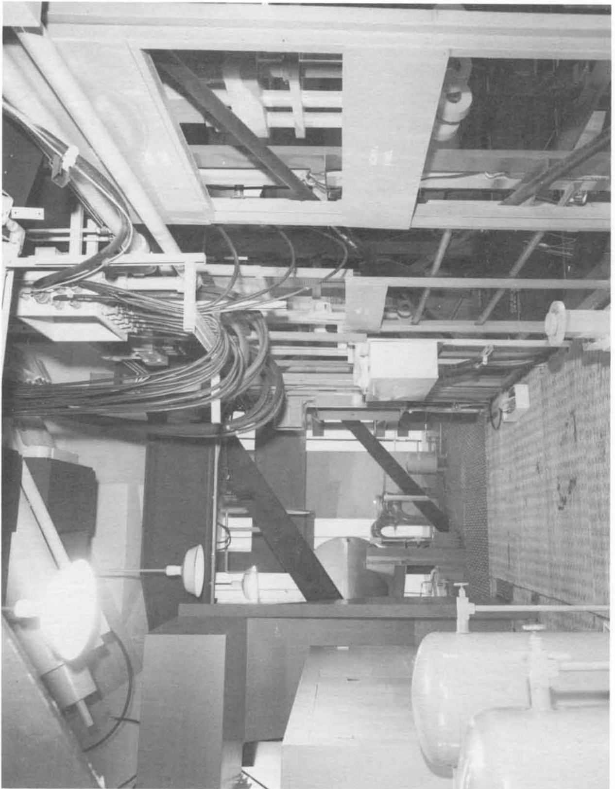
At Column K looking north--local control station (Neg. No. 68012A dated 4-26-61).
