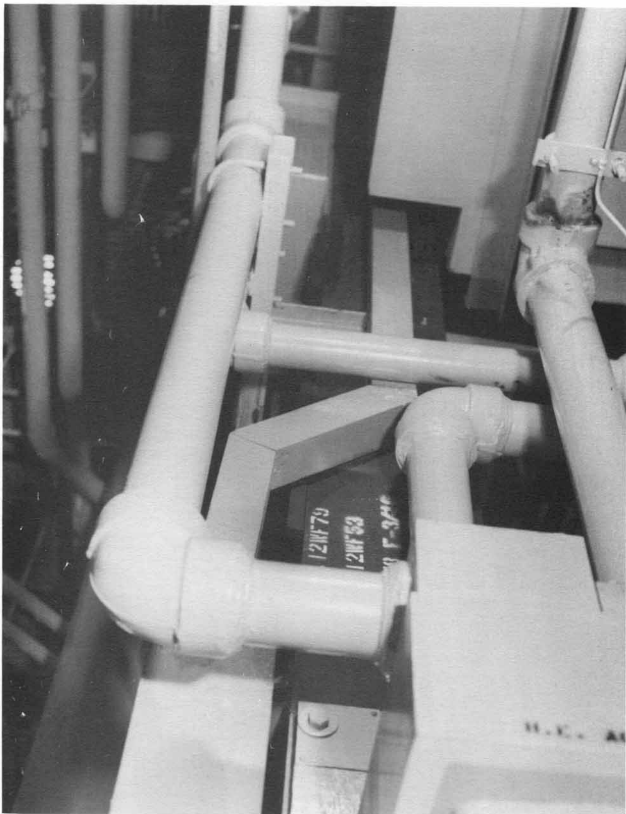
Hydraulic pipes at Column K, looking north and up (Neg. No. 66650A dated 4-3-61).
