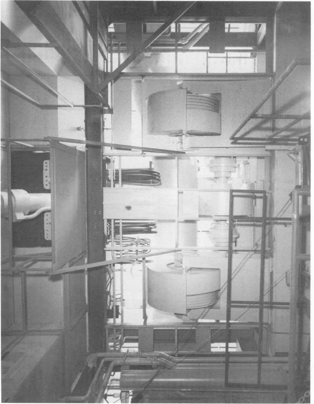
Drive mechanism at Column J to K, looking east (Neg. No. 68016A dated 4-26-61).
