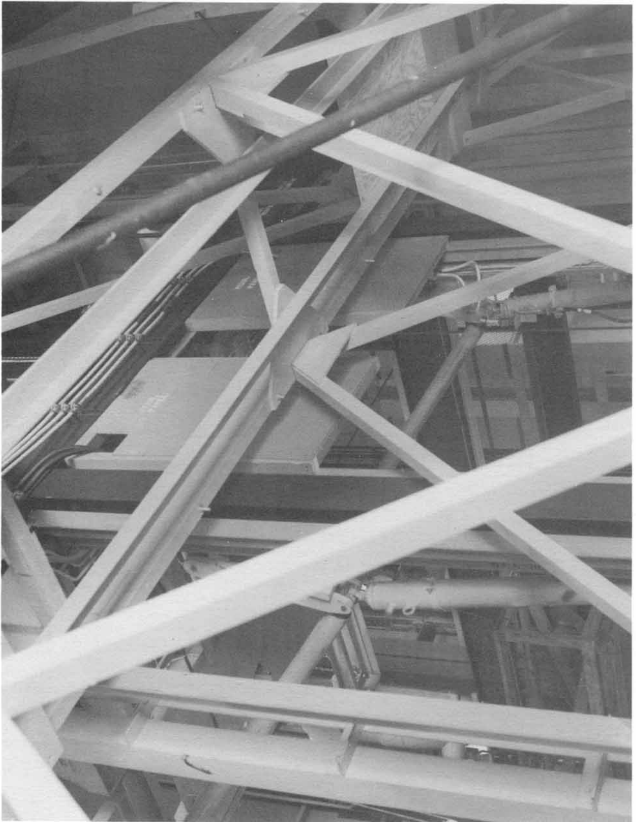
Looking from Column B past counterweight to missile enclosure steel (Neg. No. 68028A dated 4-26-61).
