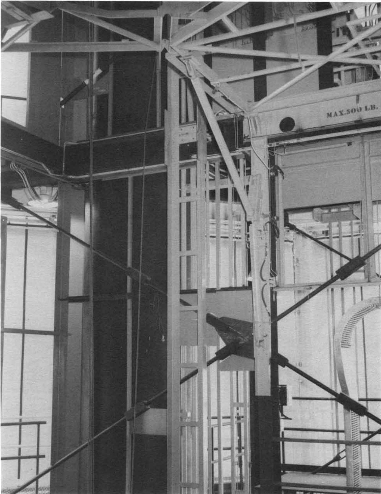
Looking south to work platform tubing from Column J (Neg. No. 68035A dated 4-26-61).
