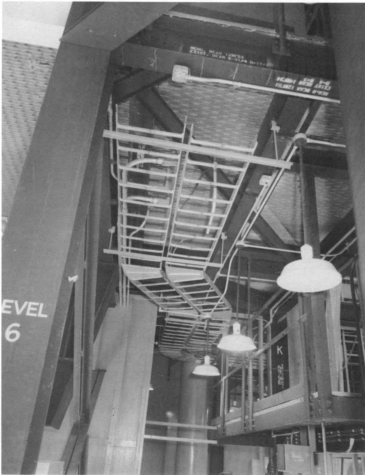
Looking up and west from near Column D (Neg. No. 68077A dated 4-27-61).
