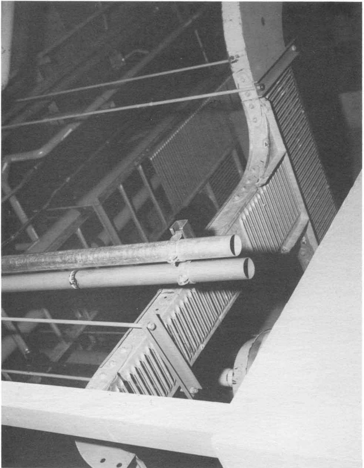
Showing proper routing of facility cable tray and conduit above nonessential and essential bus (Neg. No. 67561A dated 4-19-61).
