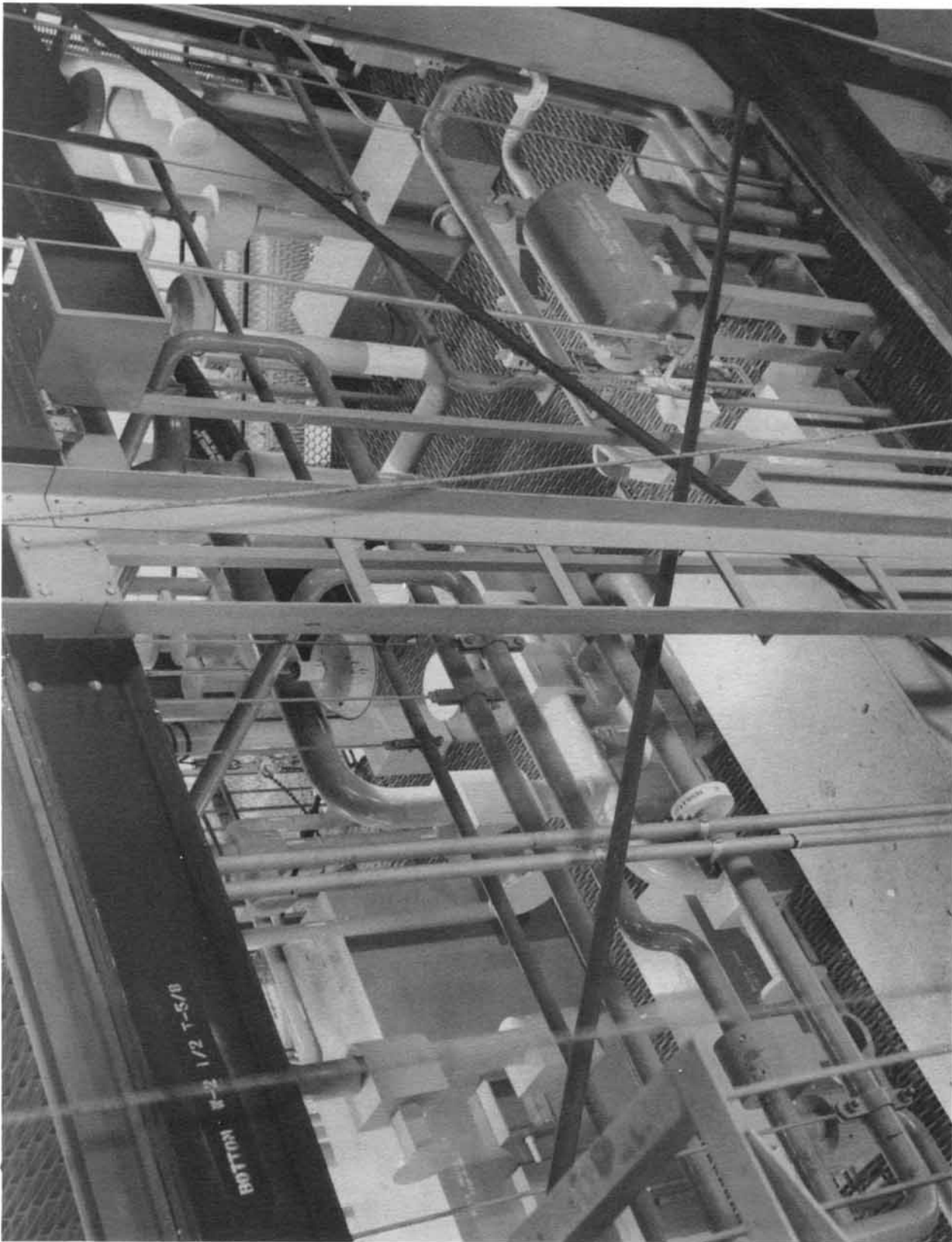
Looking from south side down to Level 4 toward Column J (Neg. No. 68037A dated 4-26-61).
