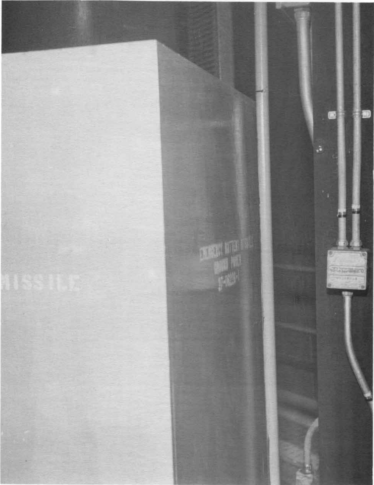
Emergency battery and water pipe (Neg. No. 67327A dated 4-14-61).
