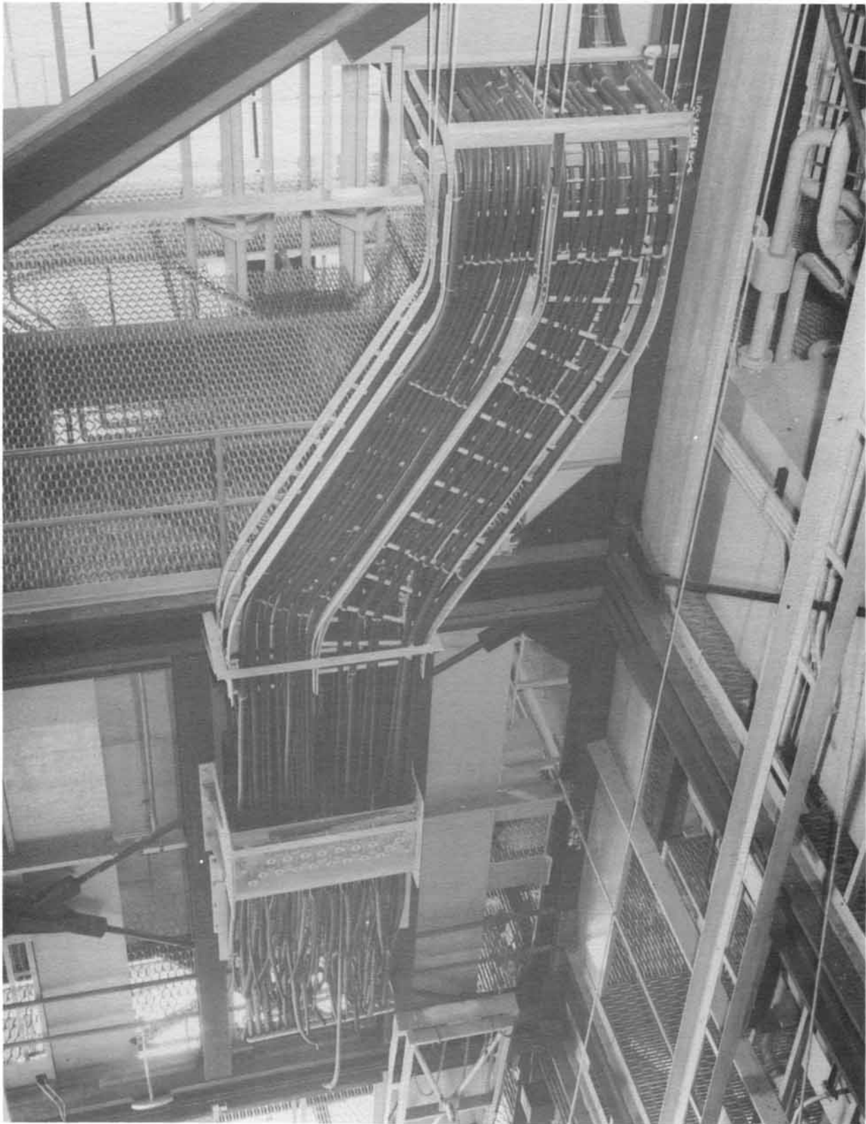
Umbilical cables from elevator (Neg. No. 68005A dated 4-26-61).
